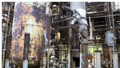
Water Ingress: Toxic Cloud & Groundwater Contamination
